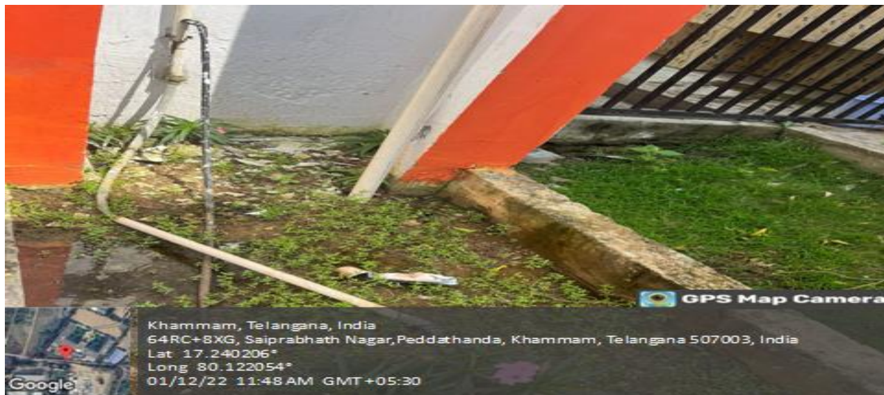
Fig 15: RO water pipelines
