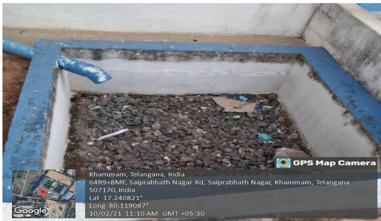
Fig 1: Rain Water Harvesting Pit
